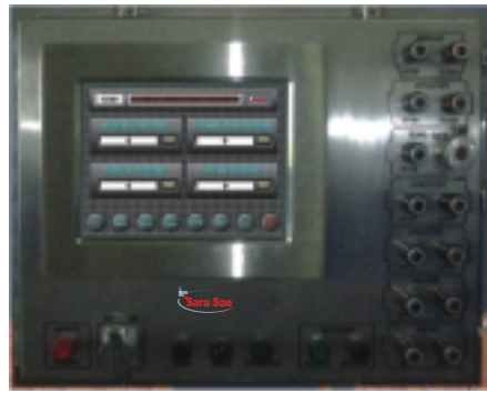
Smart Control Panel
